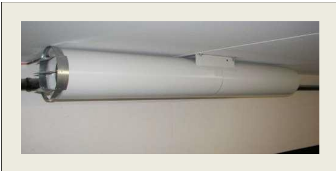
Figure 16 Car Park impulse Ventilation Fan
