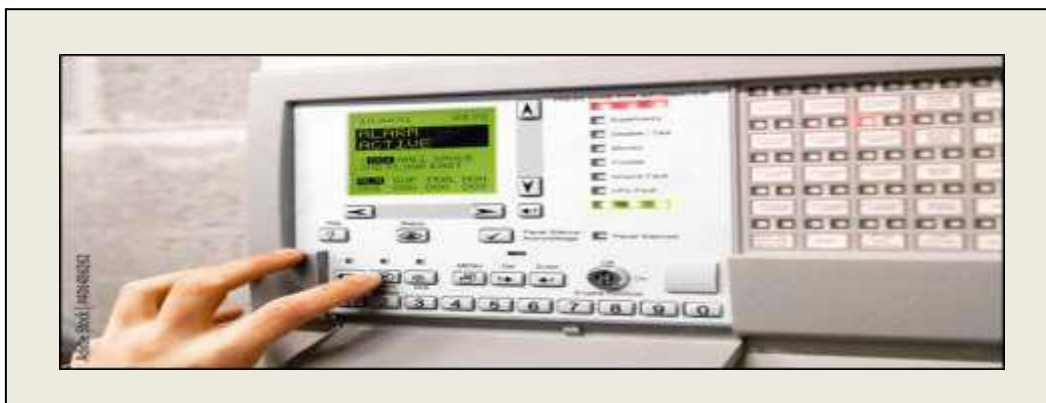
Figure 5 Fire Alarm Panel
