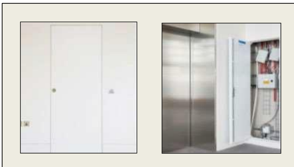
Figure 21 Service Risers in Common Areas
