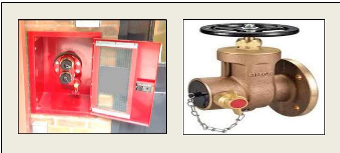
Figure 11(a) Inlet Breeching at exterior of building
