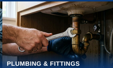
PLUMBING &amp; FITTINGS
